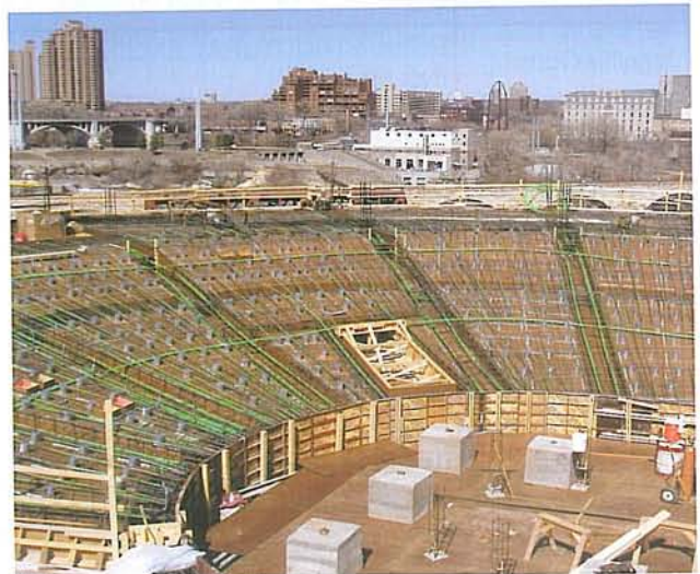
Fig. 3 – The center under construction. Note the complex layout of the radial/circular network of tendons.
